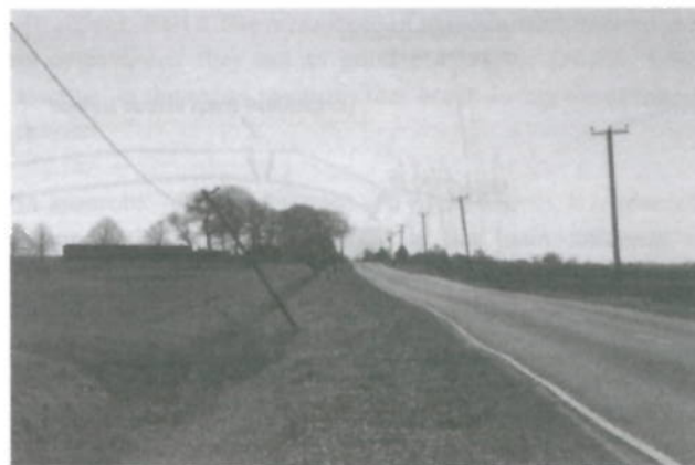
Figure 3. A section of the A1011, Bates Drove, Norfolk, showing leaning telecommunications pylon (left) and undulating road surface due to soil shrinkage
