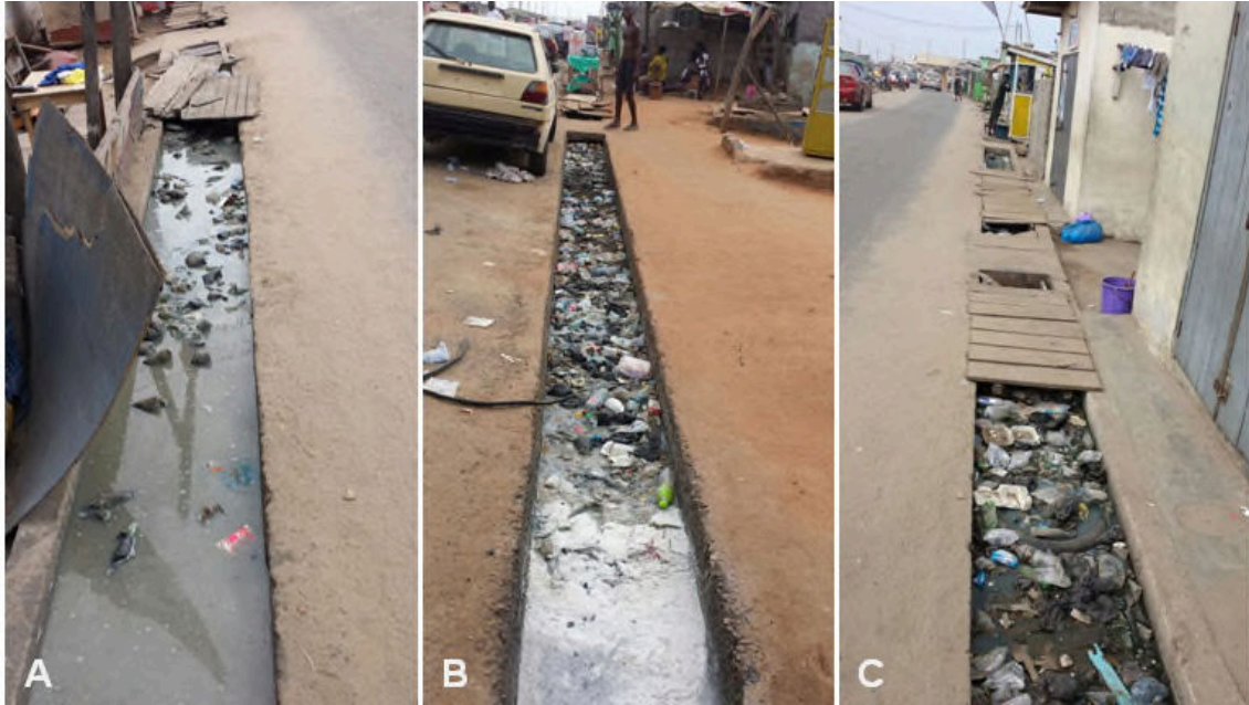
Figure 4: Choked drains in Chorkor (A) and in Shiabu (B & C)
