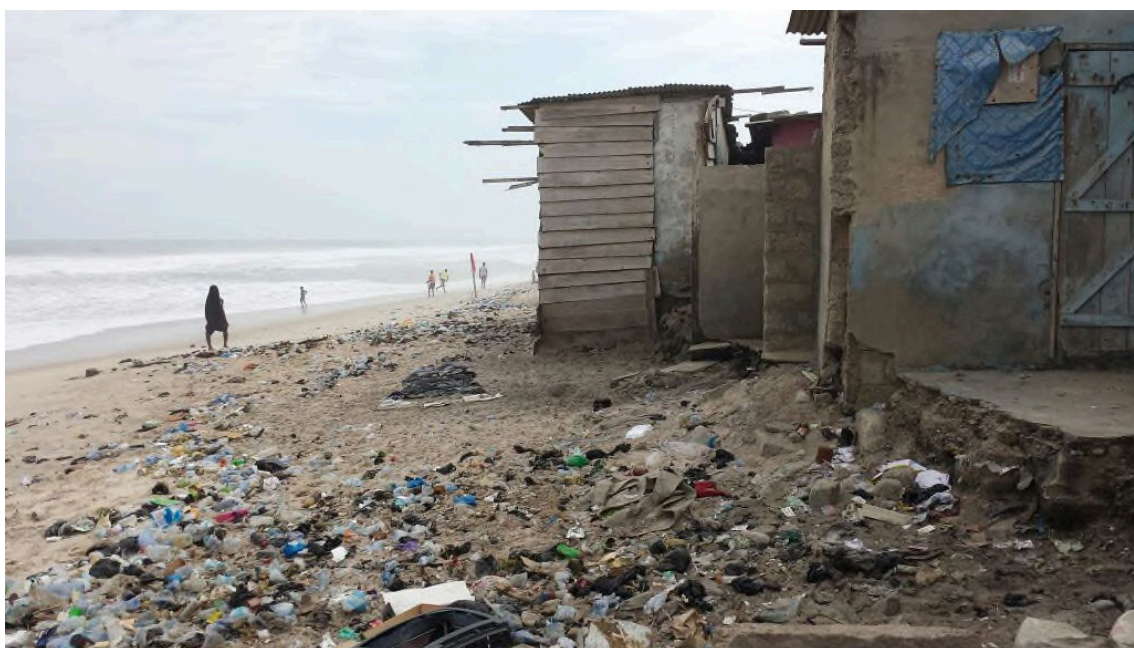
Figure 6: Foundation eroded by seawater (Shiabu)
