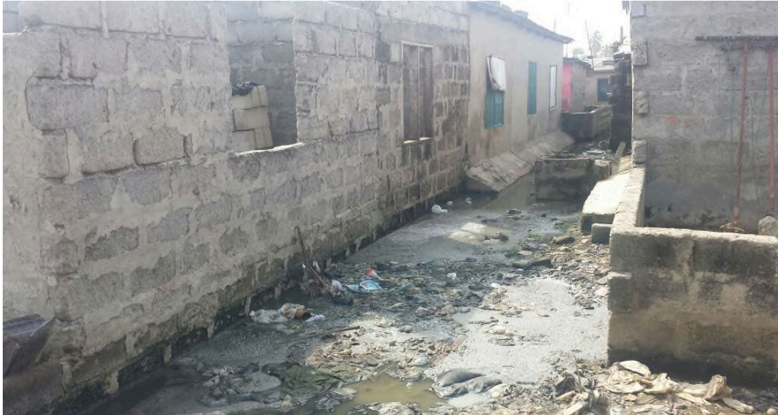
Figure 5: Sewerage from damaged sewer running between houses
