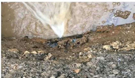
Corrosion pin hole on an iron pipe.
