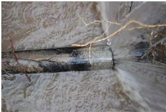
Circumferential break on an asbestos cement pipe.
