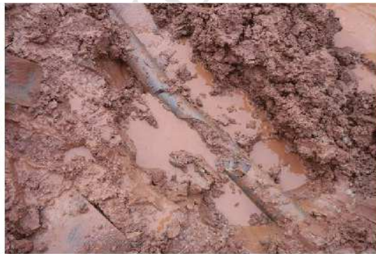
Longitudinal split on a polyvinyl chloride pipe.
