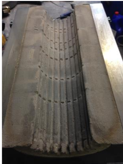
Figure_Apx D-6: Removal of refractory mastic on critical parts of the furnaces
