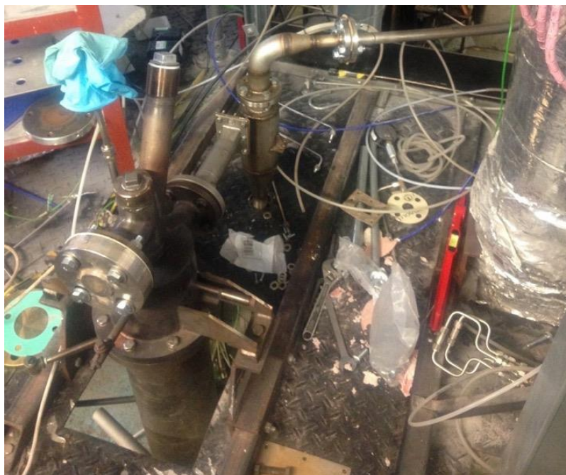
Figure_Apx C-6: New hot cyclone being installed at the exit of the calciner to collect fines carried-over from the bubbling-fluidised-bed reactor
