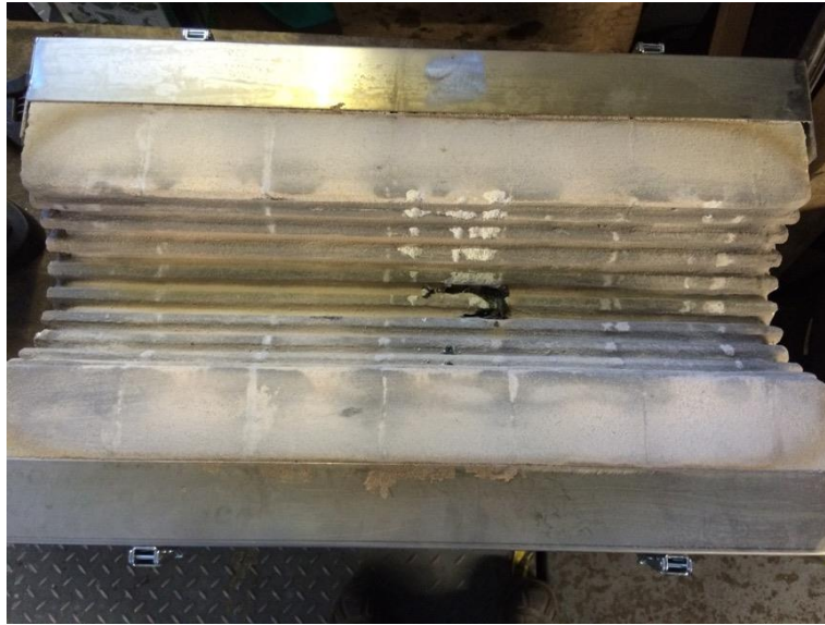
Figure_Apx D-4: Damaged furnace B
