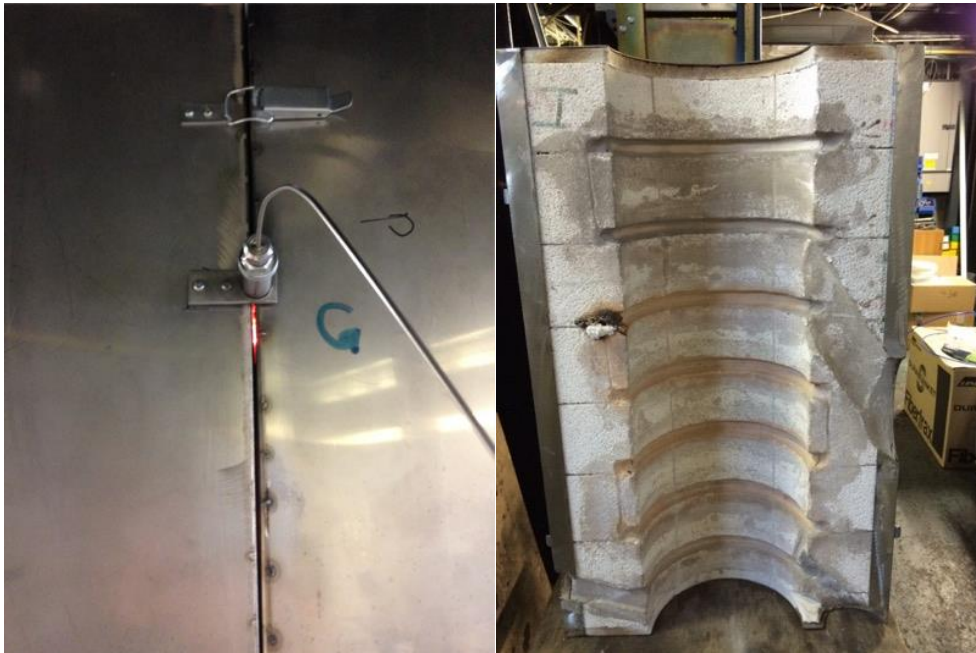
Figure_Apx D-9: The damage of heater G by electrical discharge from heating elements to the safety thermocouple
