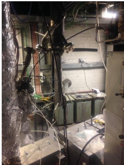
Figure_Apx C-4: Installation of the calciner with preheating line (top). Preheating line of the carbonator with installed electrical furnaces (bottom)
