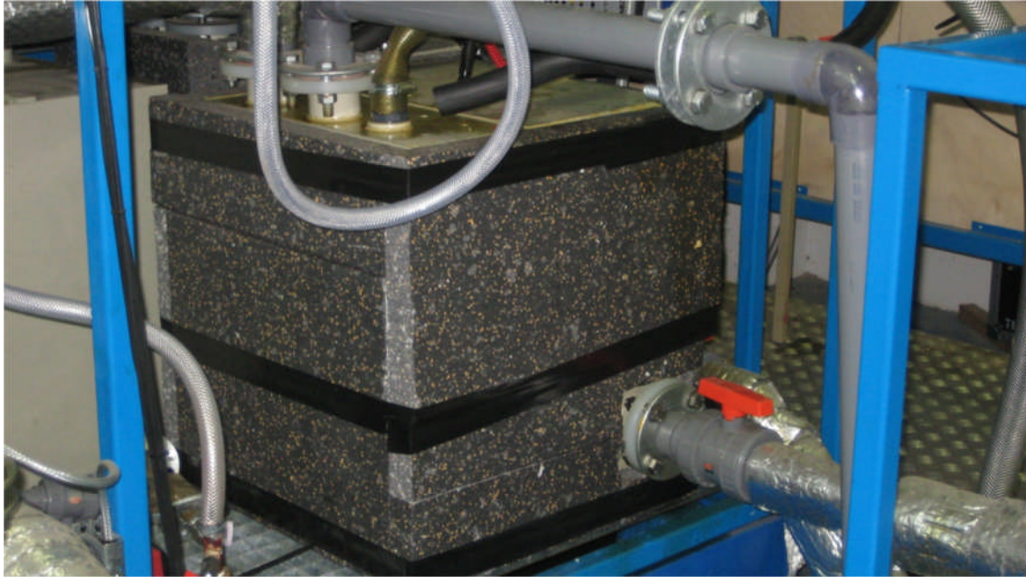
Figure 3-1: Oil storage tank
