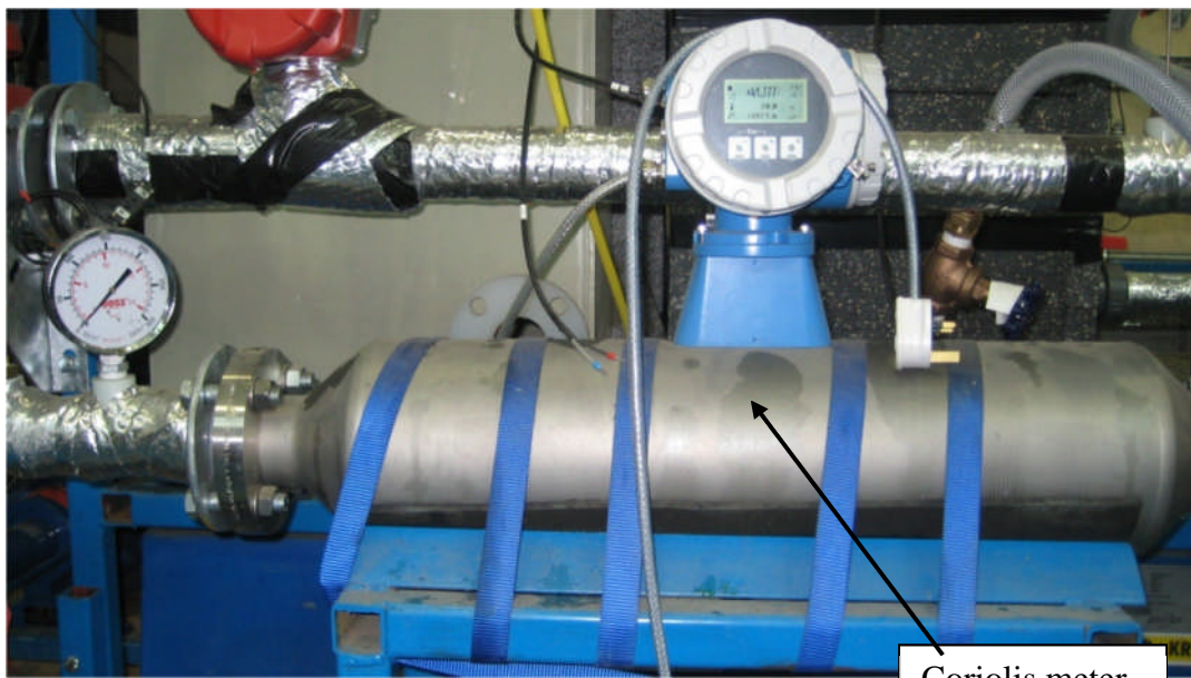
Figure 3-5: Coriolis meter and pressure gauge
