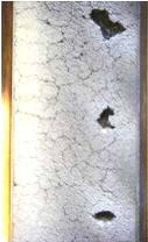
(a) Service Failure - Mudflat Cracking and Spallation
