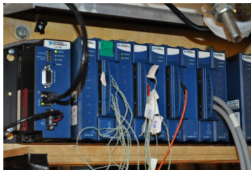
Figure 3-21 Data Acquisition Boxes (16 channels for T/C and 1 RTD)
