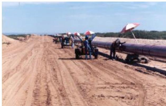
Figure 2-2: Transmission Pipeline in the Americas (Hopkins, 2002)
