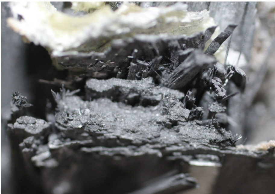
Figure 6-26 – Section of the lower spar cap illustrating significant longitudinal splitting and evidence of compressive translaminar fracture (Source: Author)
