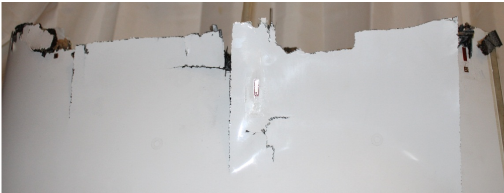
Figure 6-36 – Left wing upper surface. The impact location can be identified as a semi-circular cut-out in the top centre of the image (Source: Author)
