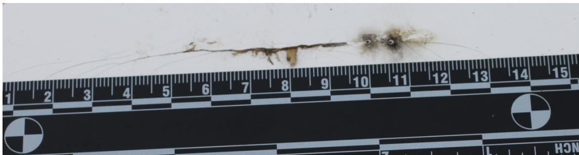
Figure 6-4 – Span-wise crack showing evidence of arcing damage (Source: Author)
