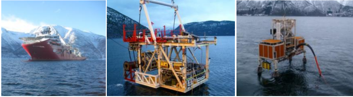
Figure 1-3: Picture of Trial vessel, Submersible Remote Pipeline Repair and Hot Tap welding equipment 8
