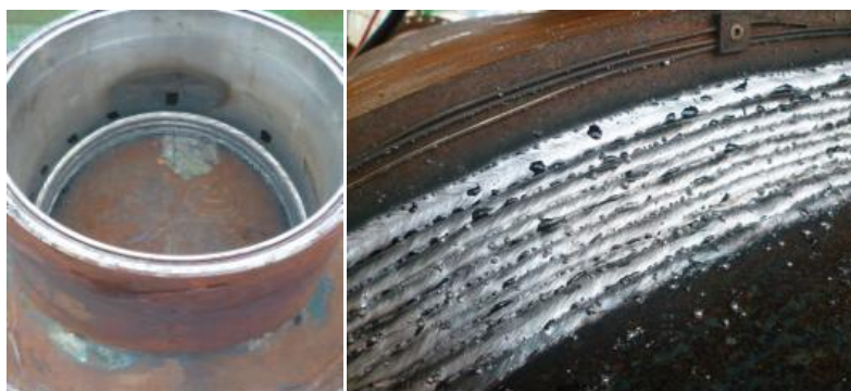
Figure 2-21: 3-Pass retrofit Tee fillet weld for remote hot tapping and 59-pass sleeve repair weld 105
