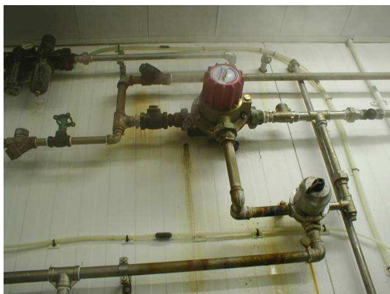
Figure 11: Example of water pipework
