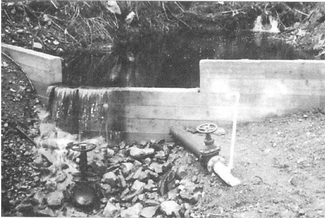
Figure 46 Example of an intake design with concrete weir, embedded penstock, and drainage pipe (Smith and Maher, 2001)
