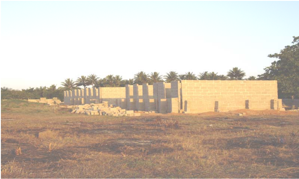
Photo 5.2: Part of the construction of Tambani Ward secondary school located at M'baya and supported by SONGAS project.
