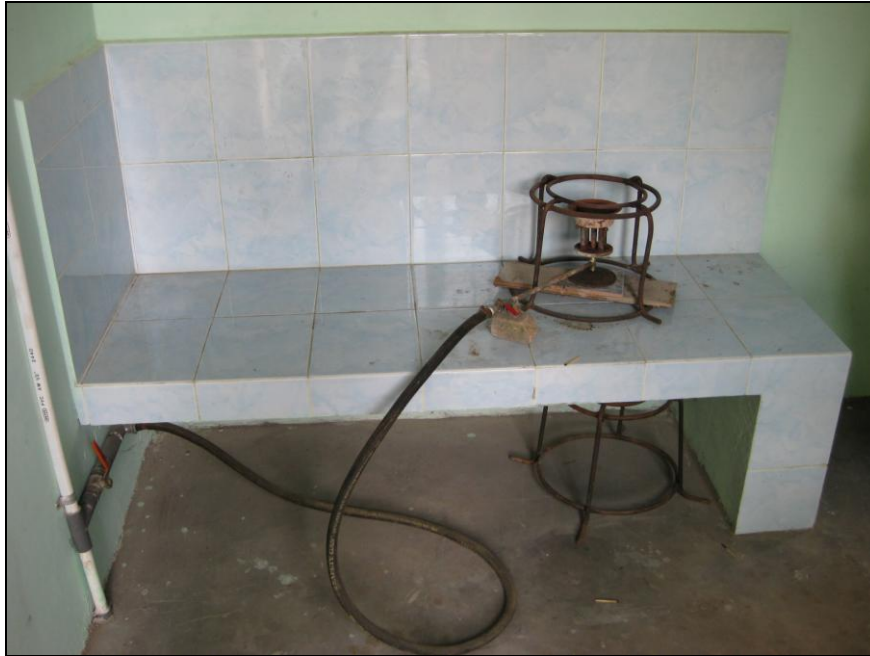
Figure 3-8 A biogas plant in a sanitation centre in Java
