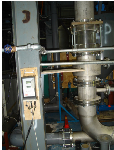
Figure 3. Photographic view of return path to riser base (downcomer).
