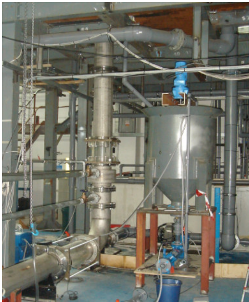
Figure 2. Photographic view of horizontal pipeline-riser base along with return path to sump and also return path to riser base (downcomer).
