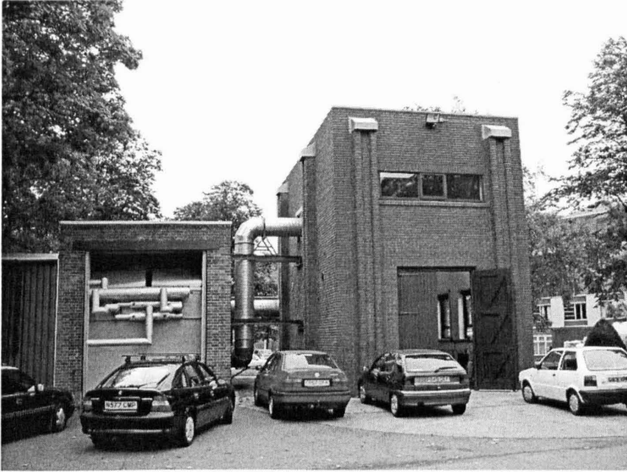
Figure 44. Tunnels and connections. The refrigeration plant can be observed on the left.
