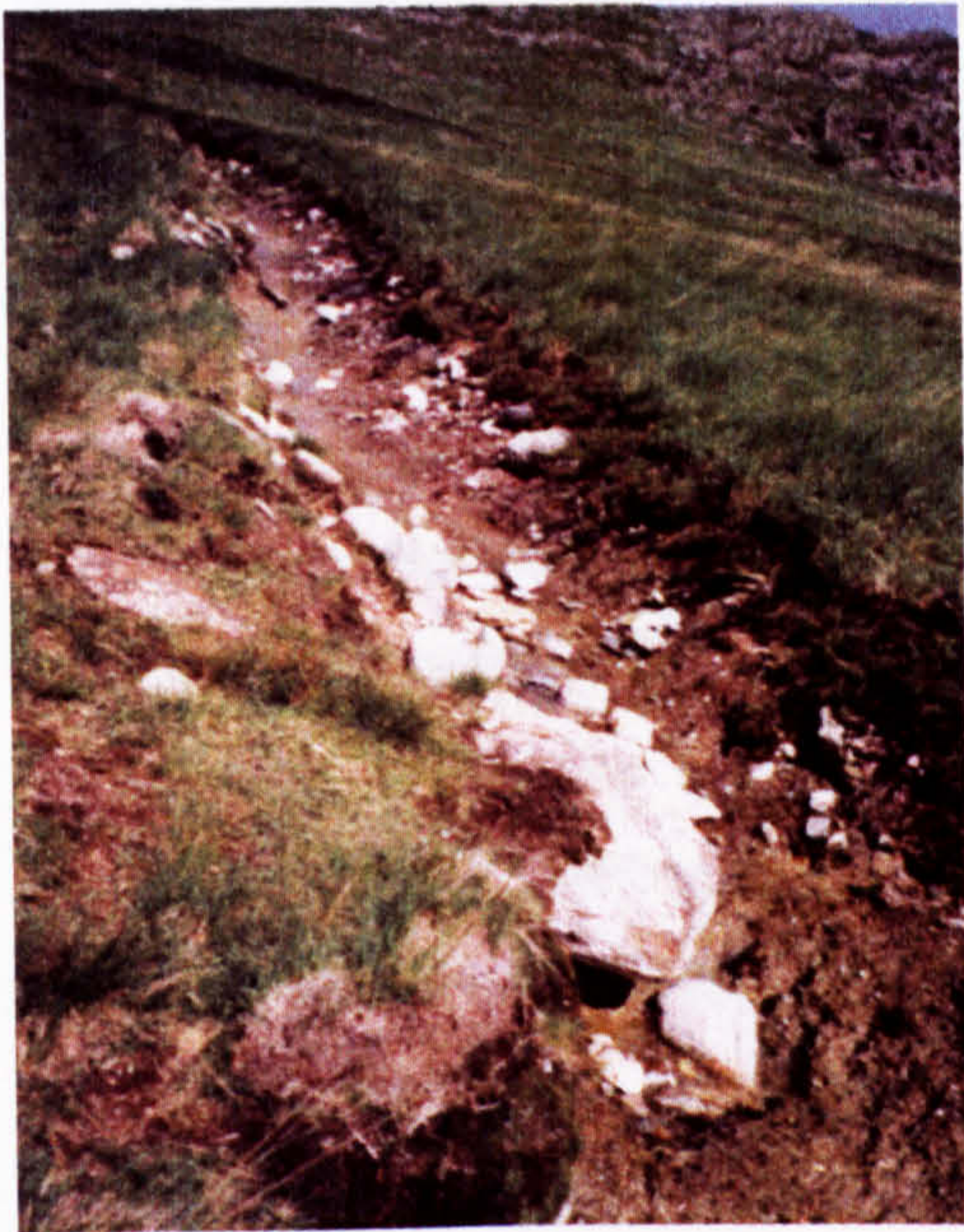
Plate 2.3 Eroding drain on marginal agricultural ground (Beddgelert, Wales).
