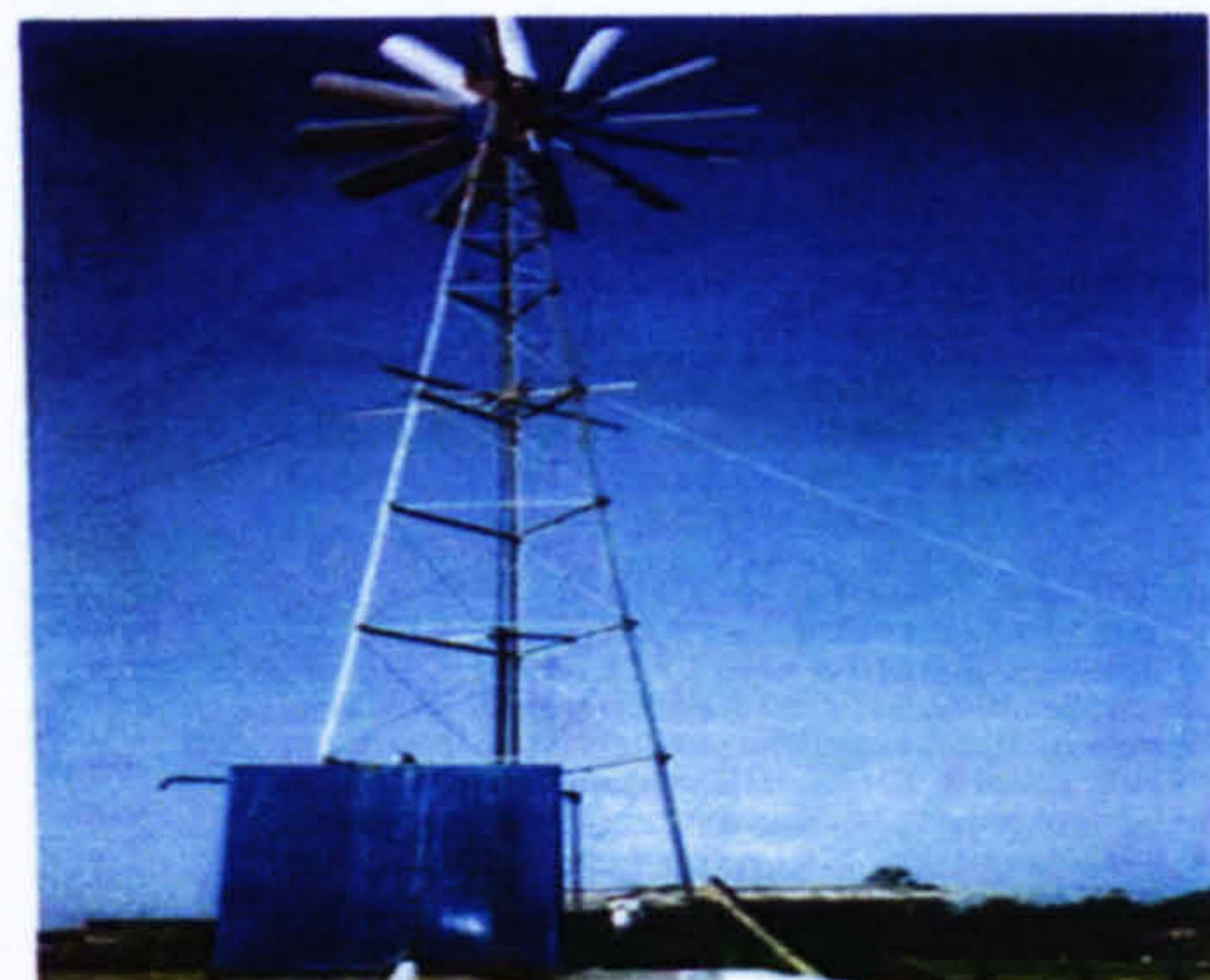
(b) A wind pump set installed by BCAS at Patenga, Chittagong
