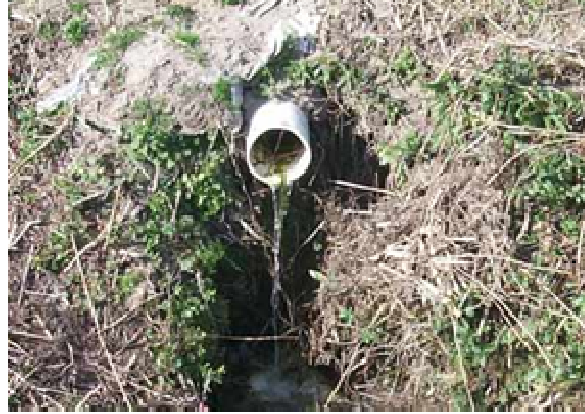
Plate 1 The outlet of an under soil perforated pipe
