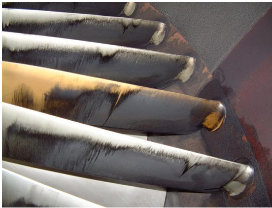
Figure 5-41 Fouling on the IGV surface from the gas turbine of Inchon Power Plant, South Korea.
