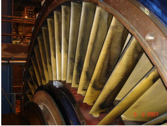
Figure 5-43 Fouling found on the IGV suction surface (Didcot Power Plant, UK).
