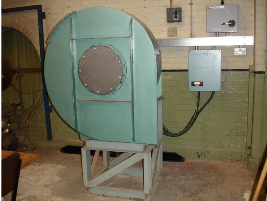
Figure 3-13 Electro-mechanical installation of the centrifugal fan model Carten Howden LTD in Test House 12.
