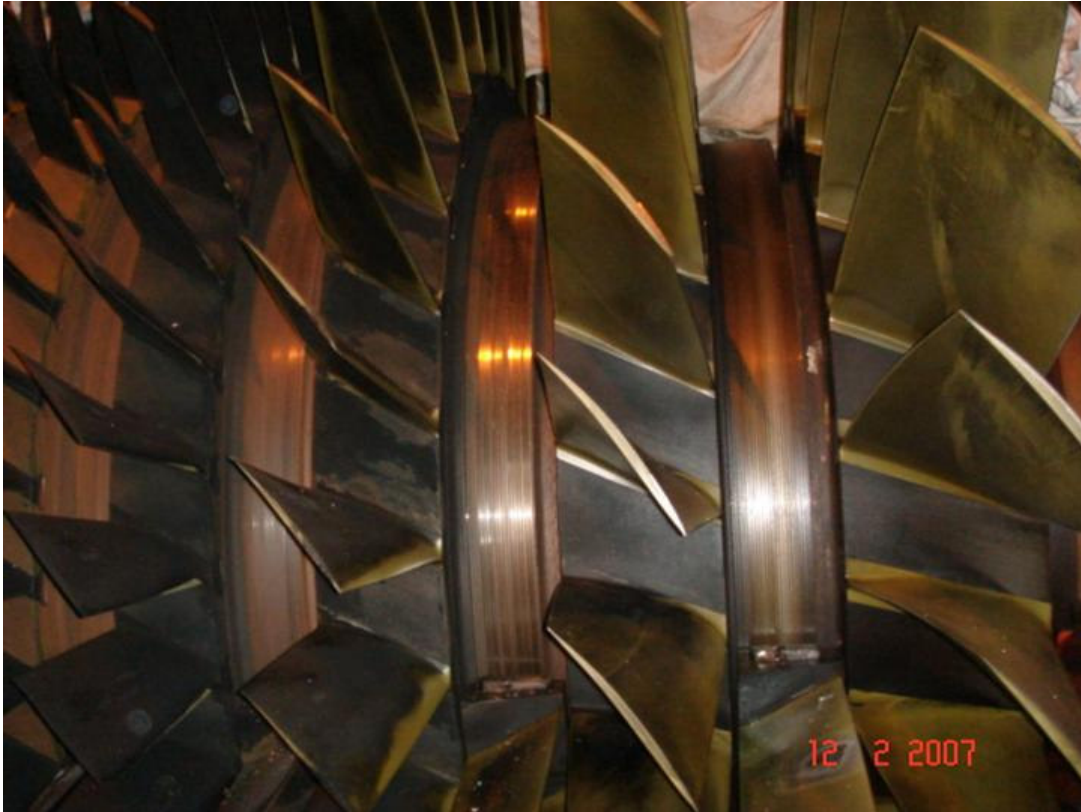
Figure 5-51 Fouling distribution on blades of the 1 st , 2 nd , 3 rd and 4 th stages (Didcot Power Plant, UK).
