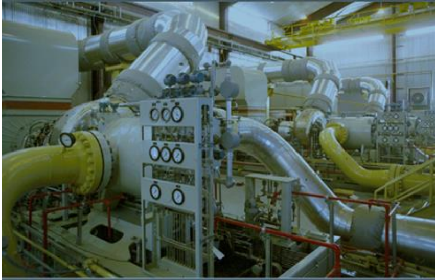
Figure 2-5 Three compressors in parallel arrangement [26]
