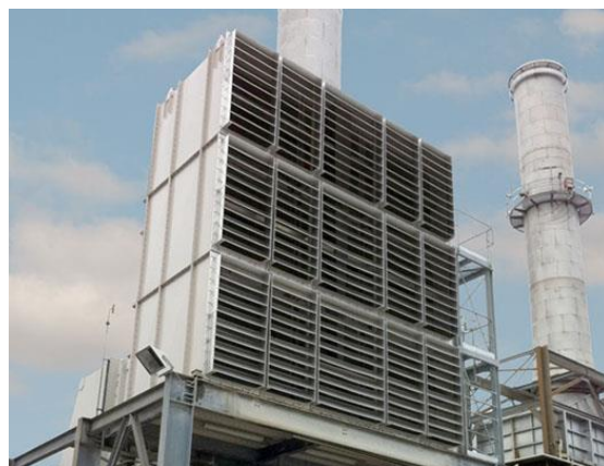
Figure 4-3 Intake filtration weather louvre (Source: Voetec, 2016)
