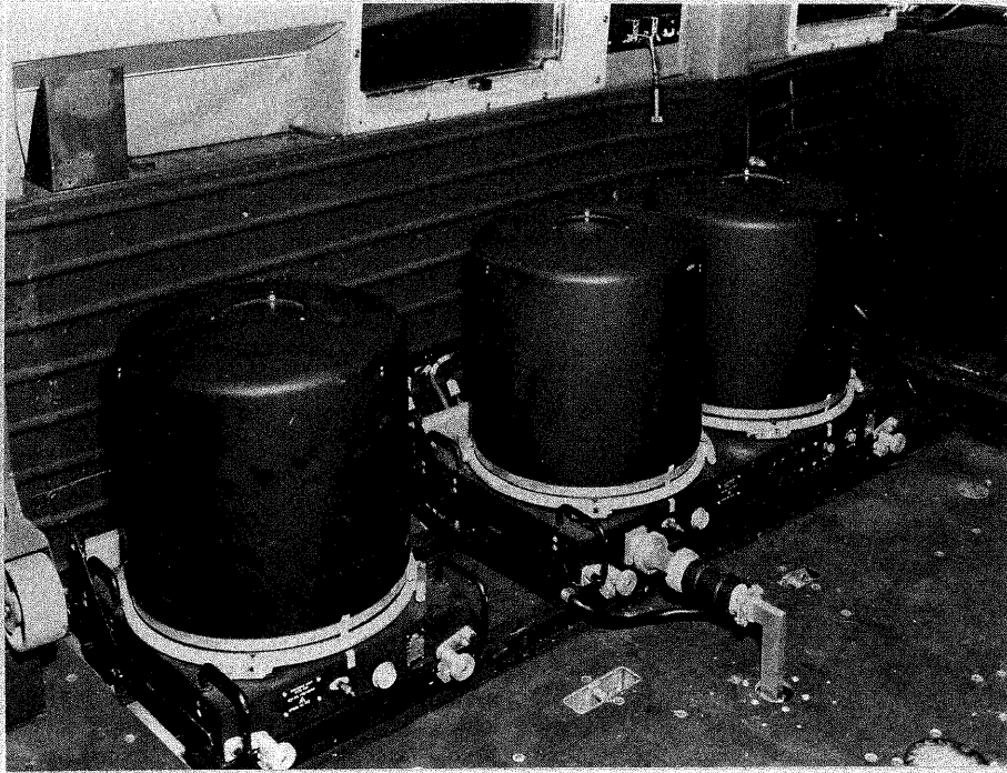
FIG. 30. DOPPLER UNITS SHOWING WAVE GUIDE PASSING THROUGH CABIN FLOOR
