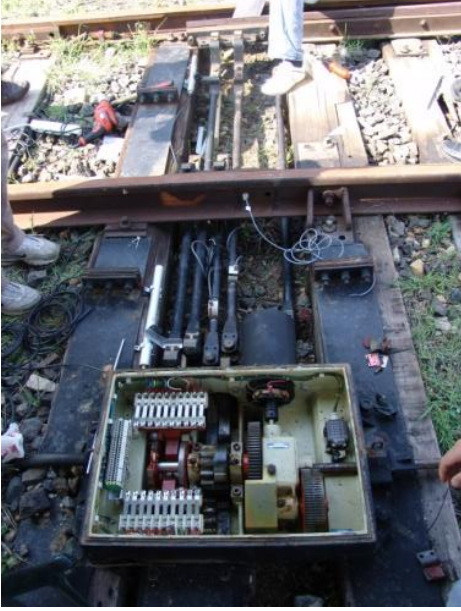
Figure 4. Electro-mechanical turnout system
