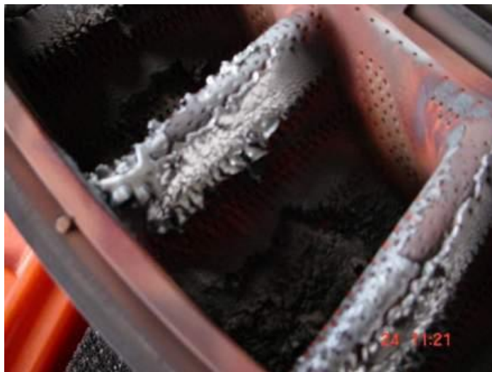
Figure 6-4: Contaminated High pressure turbine
