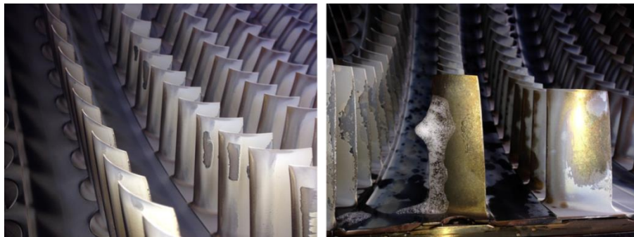
Figure 2-12: Compressor vanes before and during hand cleaning
